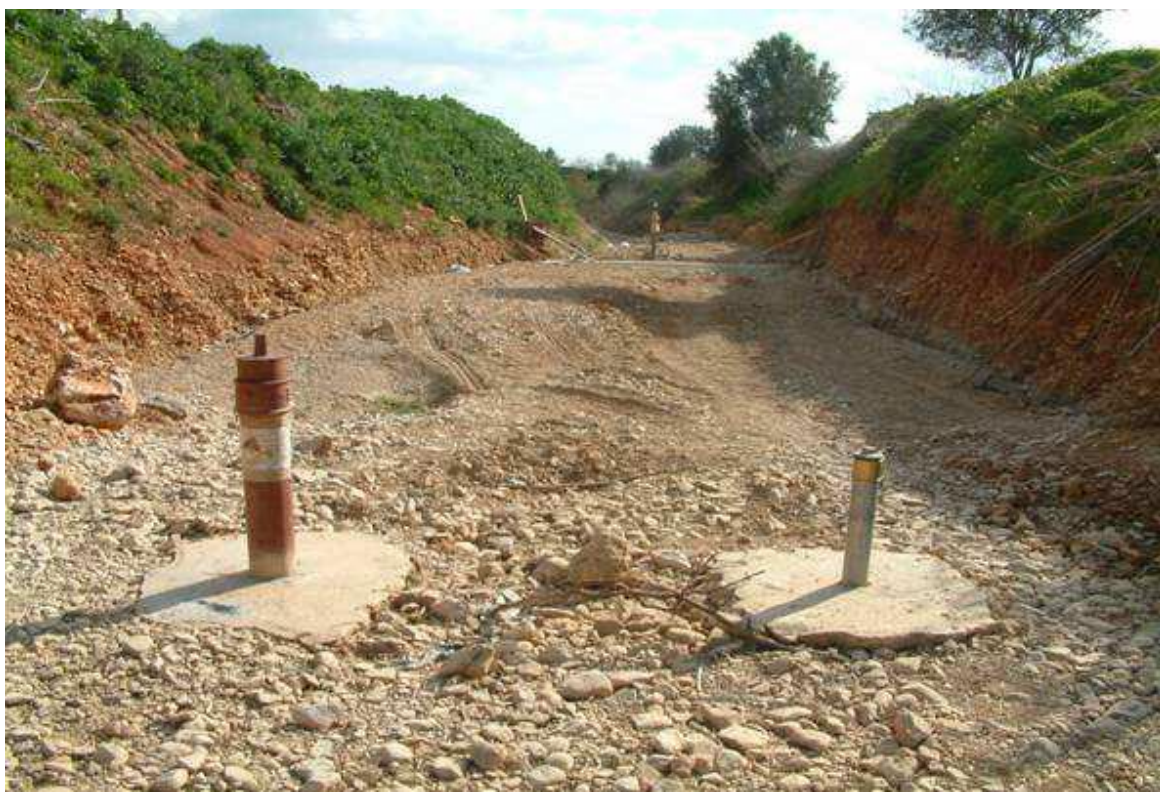
Figure 14. Artificial recharge infrastructure in the Rio Seco riverbed, constructed as part of the Gabardine Project to enhance groundwater infiltration using gravel-filled basins and monitoring wells for assessing recharge rates and water quality improvements.
